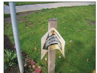
CEI teams document identified barriers in photos. These photos show the absence of safe sidewalks at a community medical center in Oregon and inadequate temporary signage.
